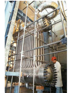
Isolation Condenser Testing
