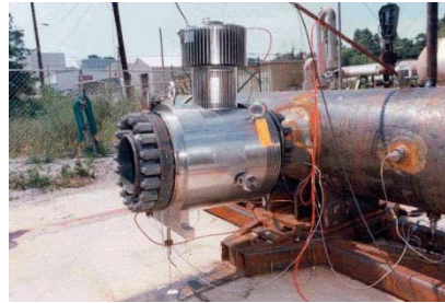
Depressurization Valve test
